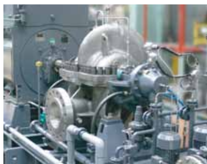
RO 1st Pass High Pressure Pump for Victorian Desalination (Australia) Pump type: MSH300/2, Delivery year: 2010 Duty: 887m 3 /h at 544m, Power: 2,000kW
